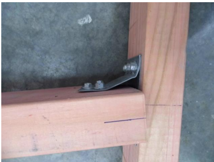
Photograph 9. Failure by bracket distortion
