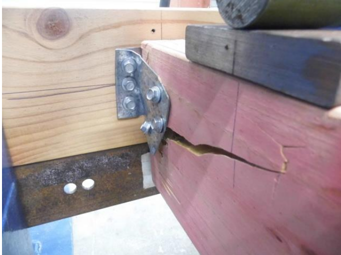
Photograph 6. Failure by end splitting
